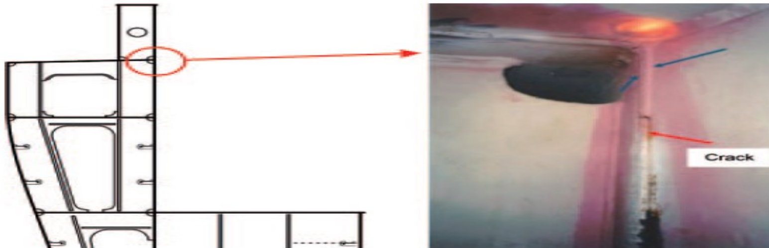
Fig. 3. Example of fatigue crack in welded joint of ship structure detail of a containership [3]
